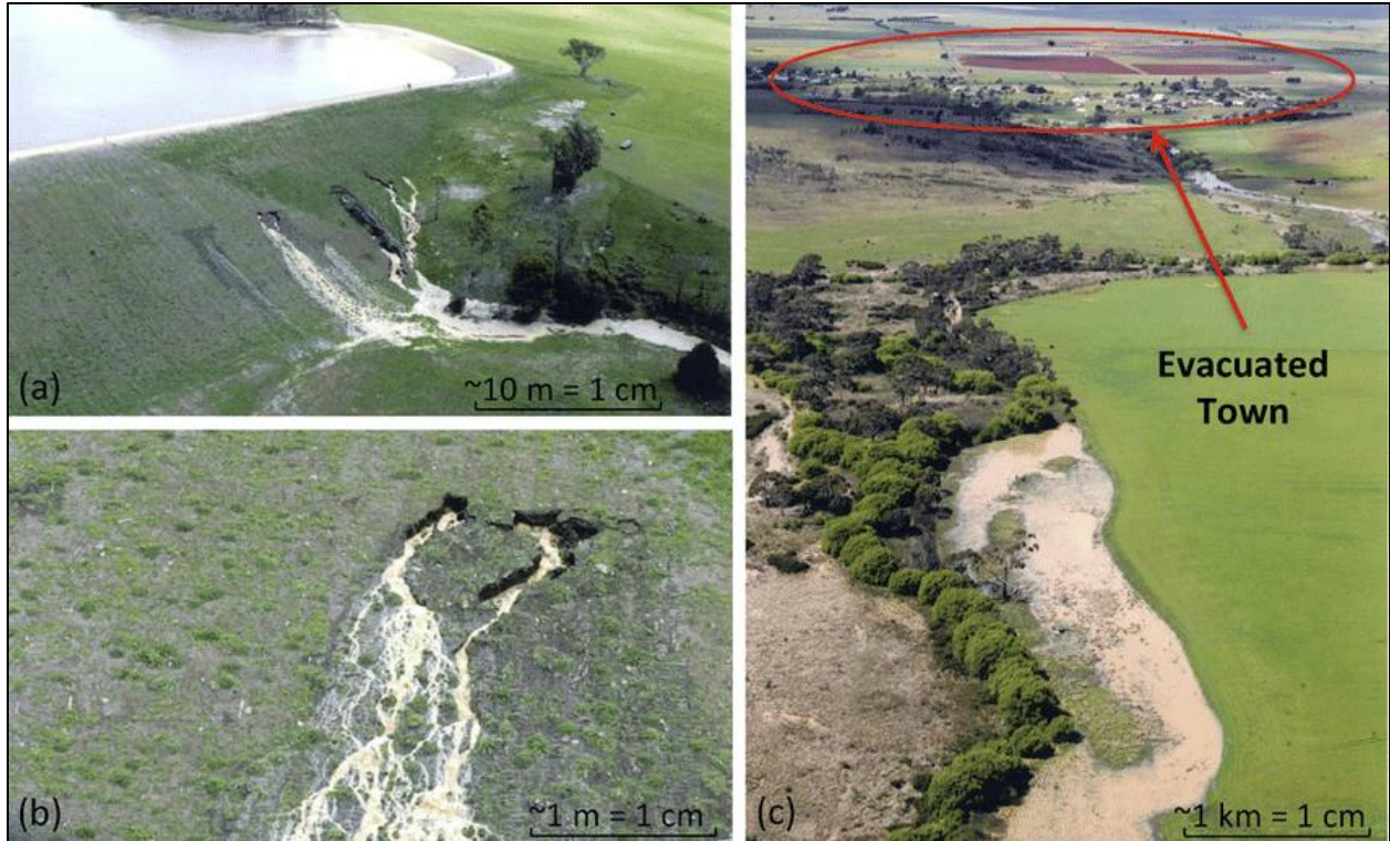
Figure 9. Internal erosion (also called piping) is a common mechanism of tailings dam failure. Internal erosion occurs when the seepage of water through the dam or its foundation is fast enough to entrain fine particles, which can lead to a loss of structural integrity, followed by a breach of the dam. The photos show the failure by internal erosion of the Tunbridge dam in Tasmania, Australia, in 2005. Figure from Fisher et al. (2017).
