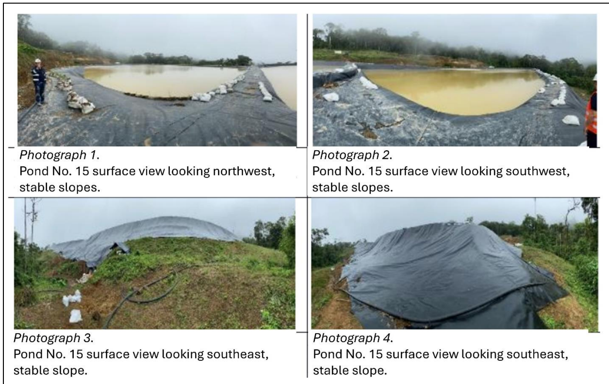
Figure 24. MAATE (2023b) states that the slopes of Pond No. 15 are stable without giving any evidence or explaining how the word “stable” is to be understood. The photos (especially the upper right) clarify that the embankments are very steep and on the order of 1V:1H (45°), which is the maximum critical angle necessary to avoid failure by internal erosion. By contrast, the U.S. Army Corps of Engineers requires slope angles no greater than 1V:5H (11° from the horizontal) to avoid failure by internal erosion (USACE, 2000). Since there are two views to the southeast and no view to the northeast, the directions might be mislabeled. Figure from MAATE (2023b) with overlay of English labels.
