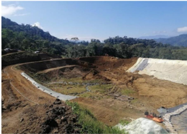
Construction of drains in the foundation of the tailings pond (file photo)
