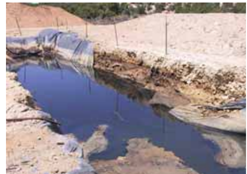
FIGURE I-8. MUD RESERVE PIT Torn liners can lead to groundwater contamination.
