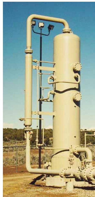
FIGURE I-12. NATURAL GAS DEHYDRATOR. Source of benzene.
