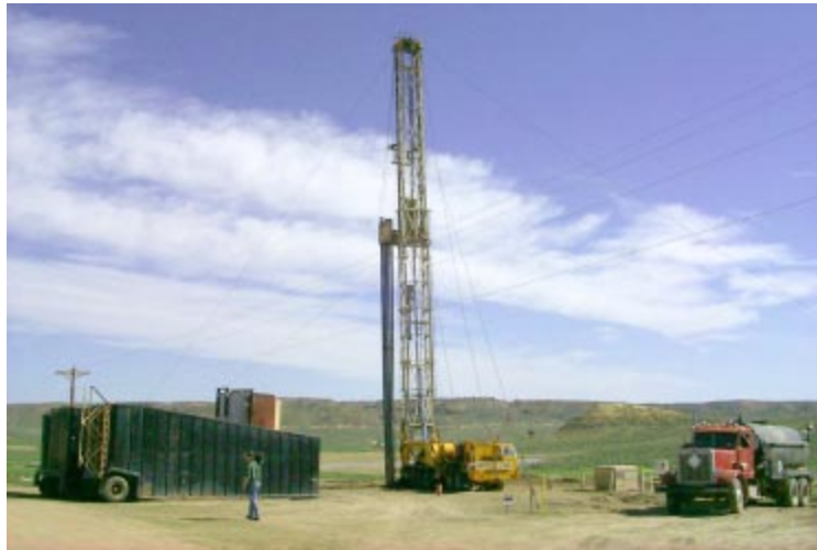
Power lines and drilling rig for CBM development in Motana's Powder River Basin.
