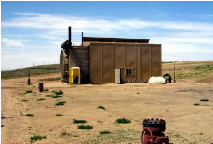
Compressor station, vegetation removal and weed infestation around Montana CBM compressor station.
