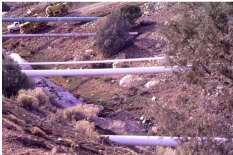
Aboveground pipelines, exposed and crossing a creek in Colorado. Note the size of the pipelines in comparison to the equipment in the background.
