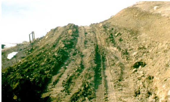
Steep topography can make surface disturbances significant: one road constructed at the Brannaman ranch to provide access.
