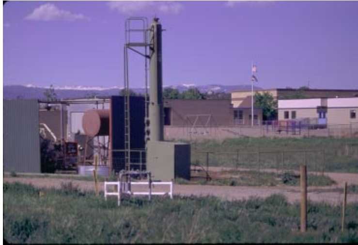
Wellhead compressor near an elementary school in Colorado.
