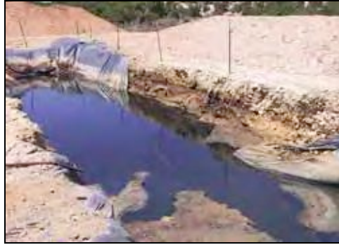
Photo of pit with a torn liner.
