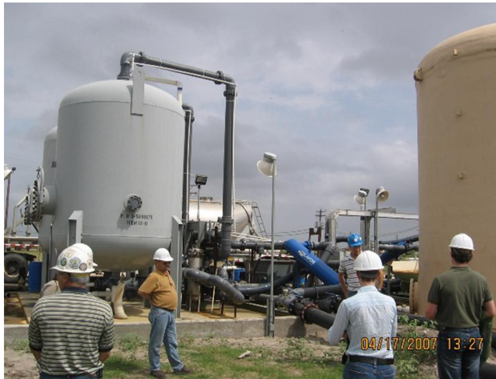
Kingsville Dome In Situ Leaching Facility in Texas. The Kingsville Dome facility was operational until 2007. Today, it is looking to restart operations. Photo source: New Mexico Mines and Minerals Division
