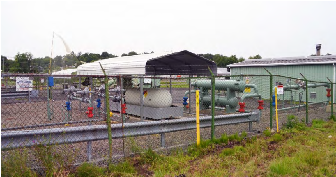
Meter and regulator station, Orange County, New York. Photo by Earthworks.
