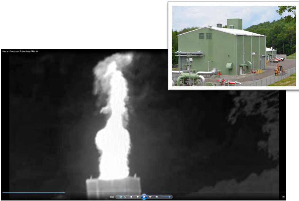
Emissions seen with optical gas imaging, Hancock Compressor Station, Sullivan County, New York. Images by Earthworks.
