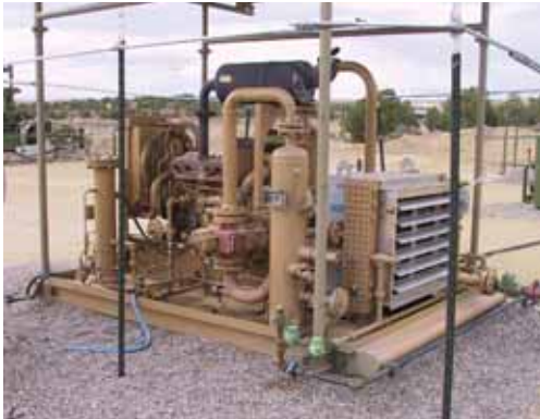
FIGURE I-14. WELLHEAD COMPRESSORS With and without sound abatement.
