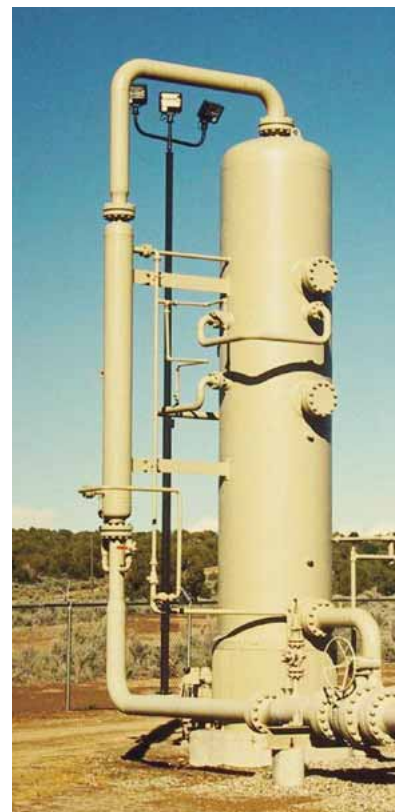
FIGURE I-12. NATURAL GAS DEHYDRATOR. Source of benzene.
