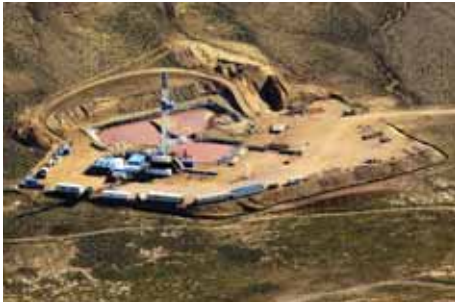
FIGURE I-36. CONVENTIONAL DRILLING SITE This site, with reserve pits disturbs 3-4 acres of land. Photo by Jonathan Selkowitz
