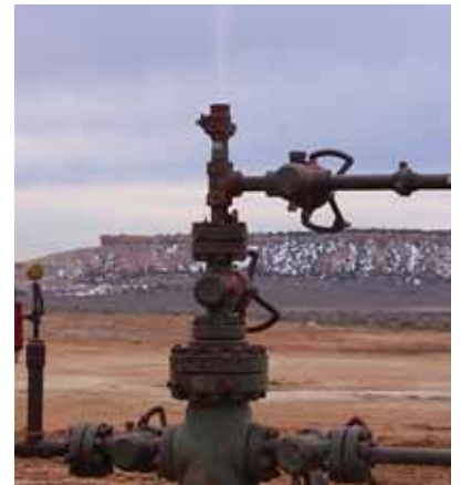
FIGURE I-29. VENTING OF GAS WELL CAN BE PIERCINGLY LOUD.
