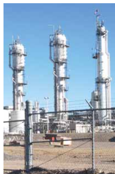
FIGURE I-13. GAS PROCESSING PLANT. Source of NO_x . Photo by Dan Randolph
