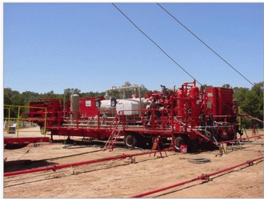
Figure 4. Example of a truck-mounted reduced emission completions (REC) unit. Photo from http://www.ipieca.org/resources/energy-efficiency-solutions/units-and-plants-practices/green-completions/ .
