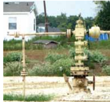
This is what a 200' setback looks like to a homeowner/landowner, and exactly how close to drinking wells these industrial activities can be.
