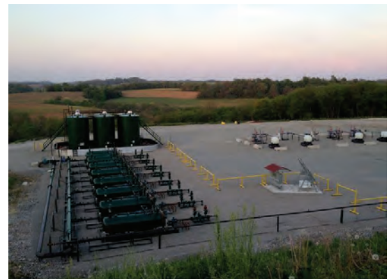
Separators split off heavy hydrocarbons from gas, and often vent methane and volatile organic compounds into the air.
