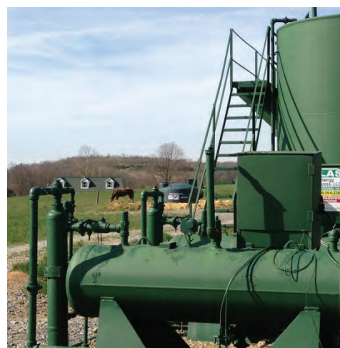
Well equipment close to home.
