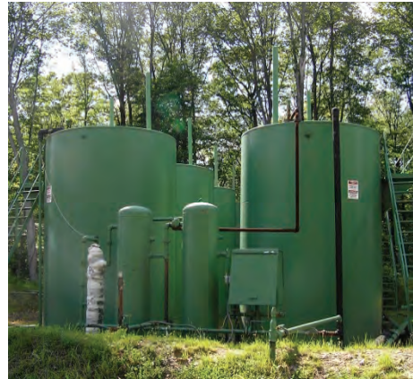
Condensate tanks pull off water from gas and can produce fumes and emissions.
