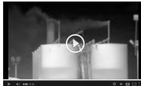
Sugarhorn facility, June 15, 2012 Infrared camera indicates extensive hydrocarbon emission. http://eaglefordreport.earthworksaction.org
