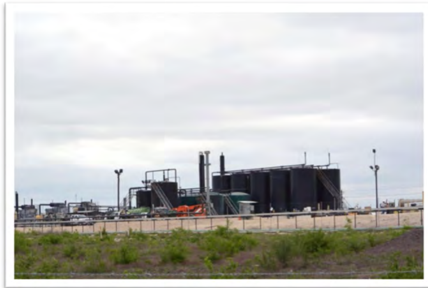
Figure 60. Marathon Sugarhorn Central Collection Facility in Karnes County as seen with the naked eye.
