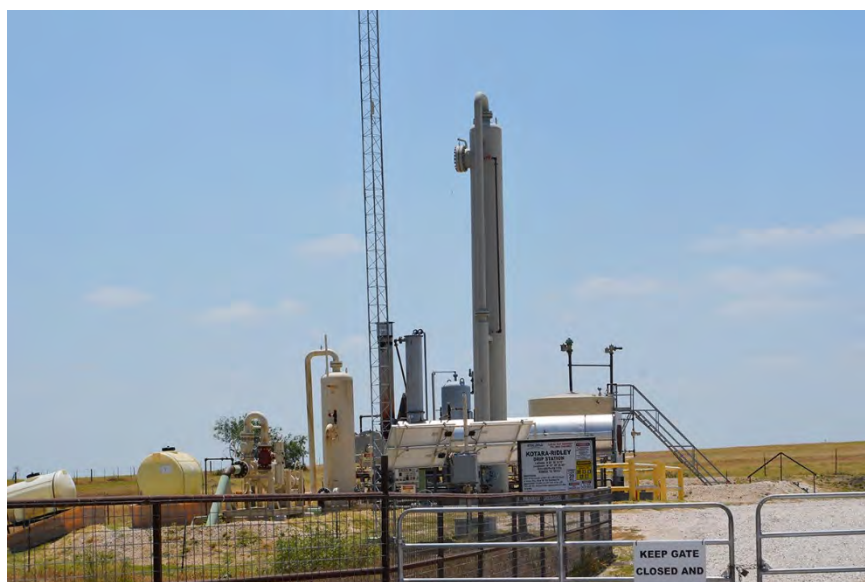
Figure 38 at right: Encana Kotara-Ridley Drip Station.
