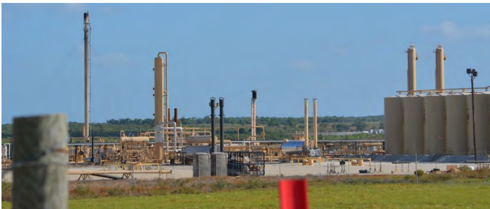
Figure 15. Marathon Sugarloaf Comingle Facility.
